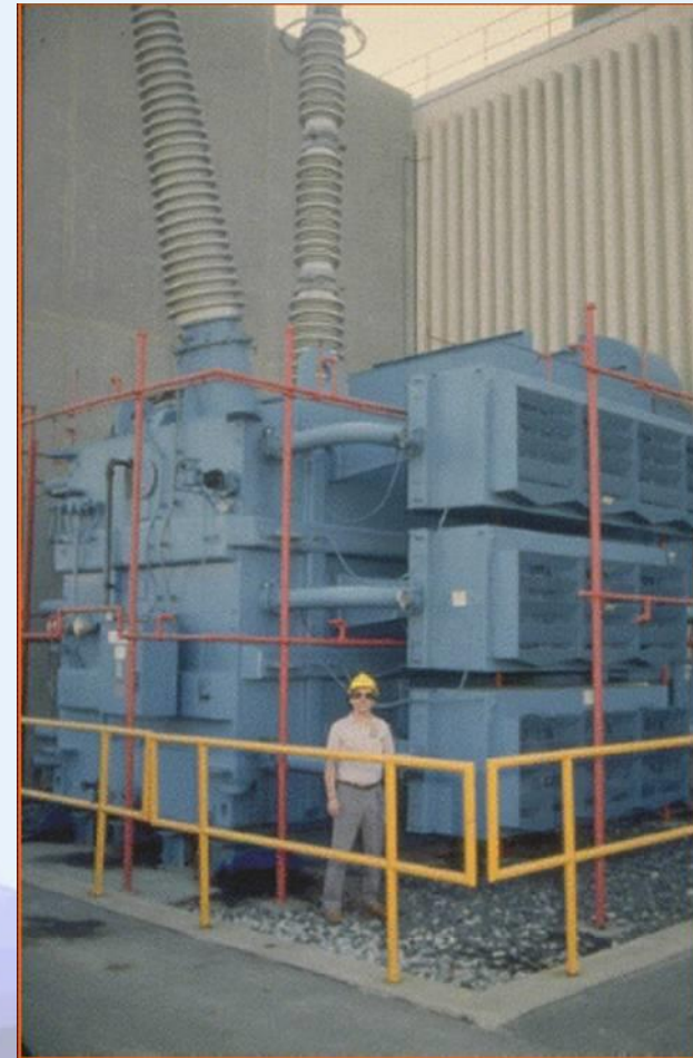
Single Phase 500 kV GSU Transformer
