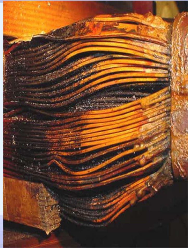
Transformer #5 Lead Overheating
