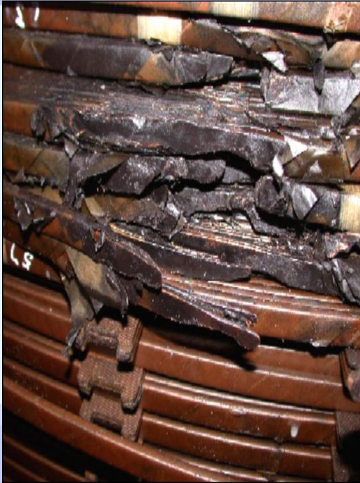
Transformer #4 HV Winding Damage
